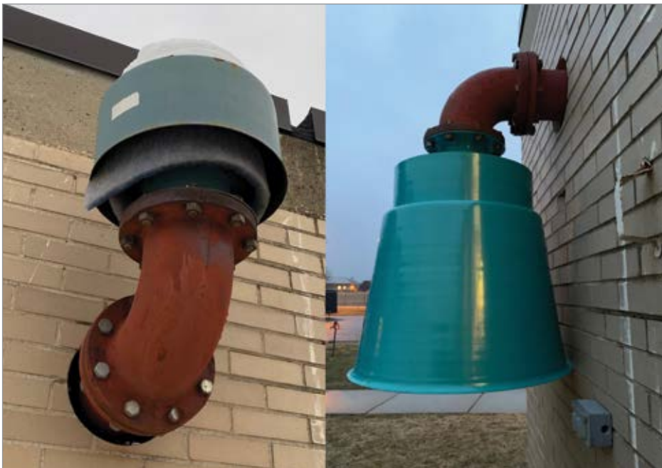
The St. Charles wastewater treatment plant reduced its energy costs and addressed safety and noise concerns by replacing the original blower inlet filter (left) for its multistage blowers with a new inlet filter silencer (right).
