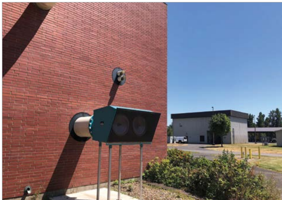
The City of Eugene installed an Endustra outlet manifold intake filter silencer at its wastewater treatment plant.
