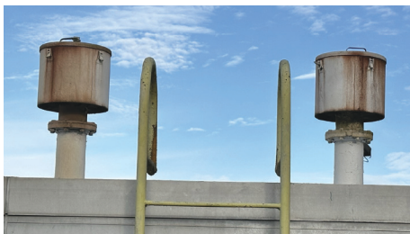
McConnellsville’s old, outdated, corroded filter canisters before the upgrade.
