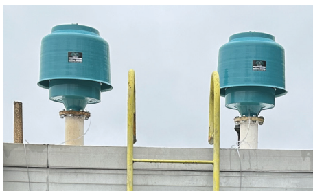
The village of McConnellsville decided to move forward. Removal of the old filters and installation of the new ones, including differential pressure gauges, was completed in one day — before lunchtime.
